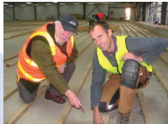
• Above: Armstrong with Dales Sports Surfaces (UK) managing director Richard Steadman during the floor installation.
